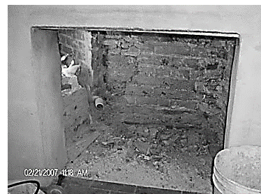
Badly Deteriorated Firebox
