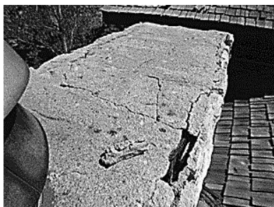
Damaged Chimney Cap
